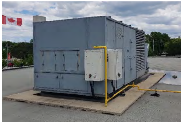
Figure 5 Multizone Packaged RTU
