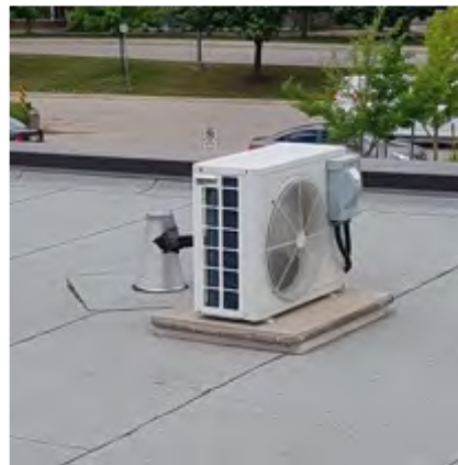
Figure 23 Mini split outdoor unit
