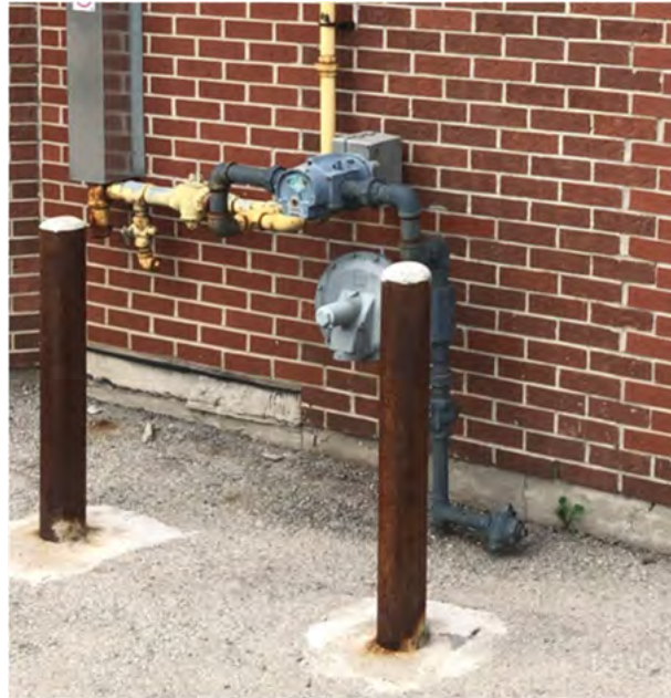
Figure 3 Natural Gas Meter
