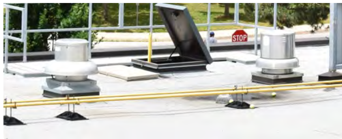
Figure 27 Kiln and Washroom Exhaust
