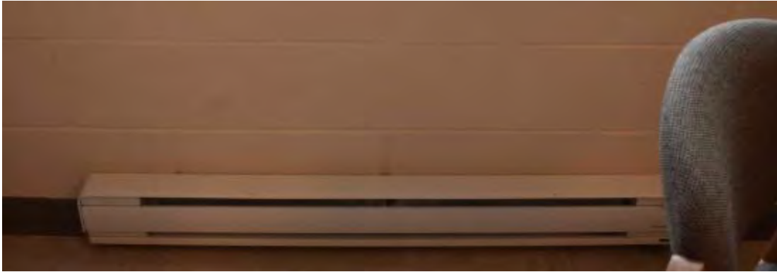
Figure 5: Electric Heater in Games Room
