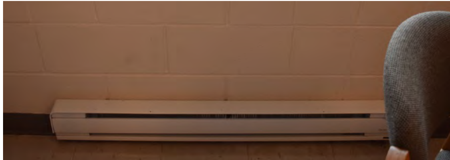
Figure 7 Electric Heater in Games Room
