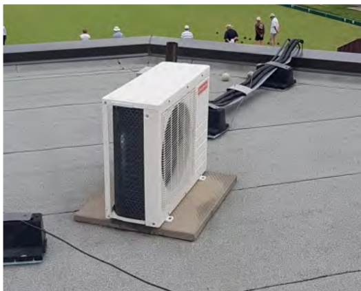
Figure 22 Mini split outdoor unit
