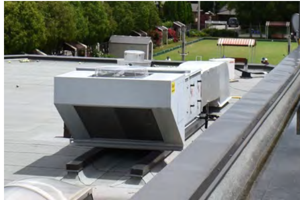
Figure 26 Kitchen Make-Up Air Unit and Exhaust Fan
